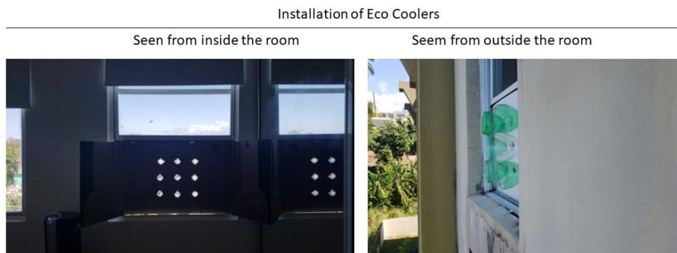
Fig. 5. Installation of the Eco Coolers seen from inside and outside of the room.
